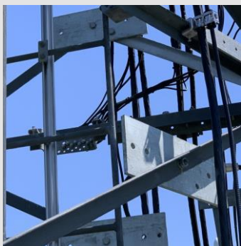
Galvanic protection of electricity pylons
