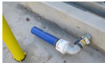
PETRO PIT 416 filter mounted on a concrete retention pit
