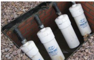
PETRO PIPE PH-616-M2 filters connected in parallel
