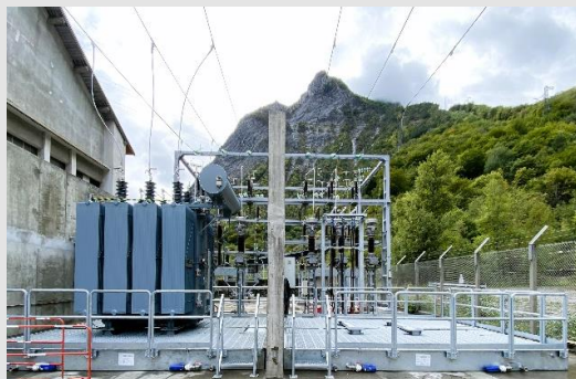
ERT-MODULO 2 tank with railing, stairs and non-slip gratings
