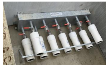
SKID PIPE for remote pit gravity drainage, approx. 200 L/min
