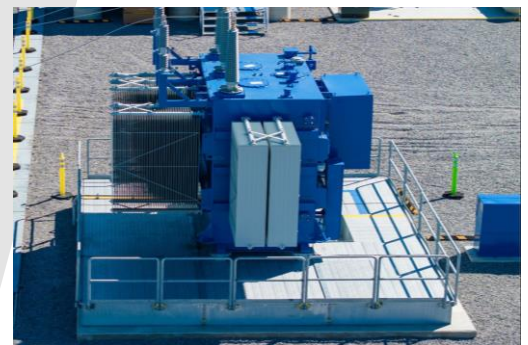
TRT-LHD-MODULO 3 retention tank with railing and access stairs for MIDEL 7131 transformer
